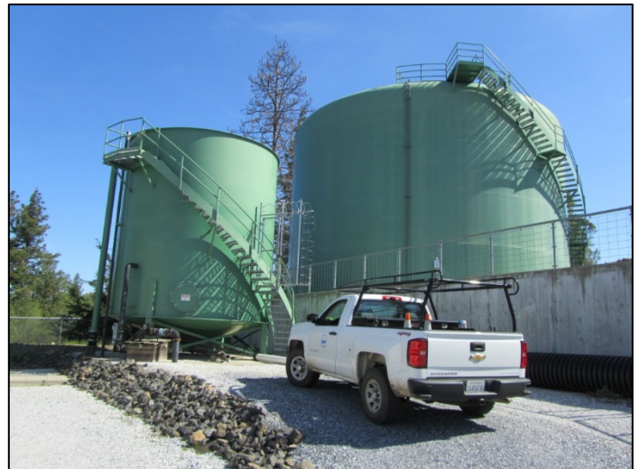
Monte Grande Water Treatment Plant - Sonora
